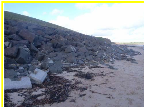
Slight flattening of profile and displaced rocks at toe of revetment.
