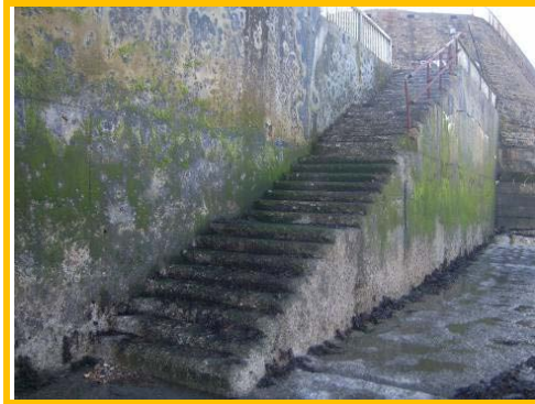
Highly abraded access steps and missing hand railing.
