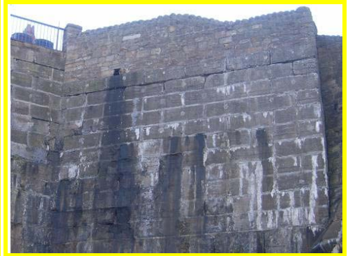
Horizontal gap in blockwork along the crest of the upper section of wall.
