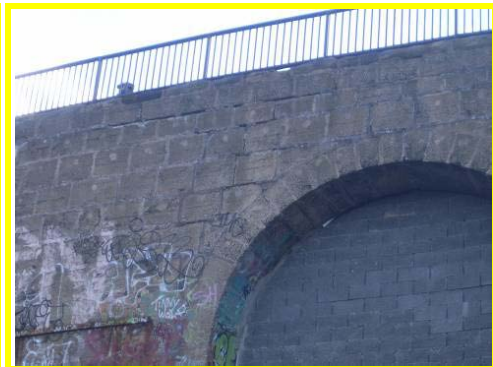
Gaps between blocks in the upper wall.
