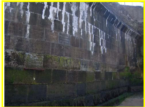
Heavy staining down face of wall.
