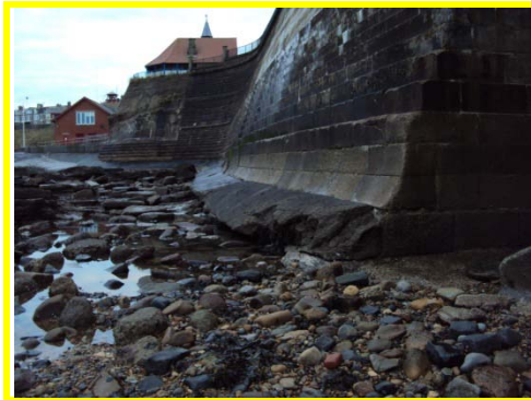
Undermined concrete apron requiring repair.
