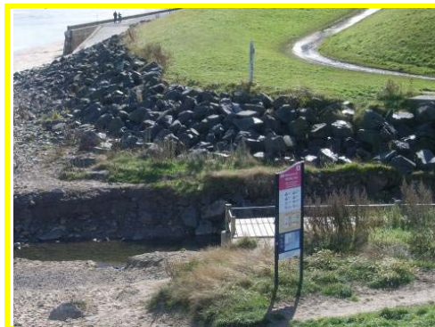
Revetment immediately south of Briardene Burn in fair condition.
