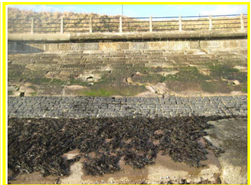
Sloping revetment with occasional cracks and mortar gaps
