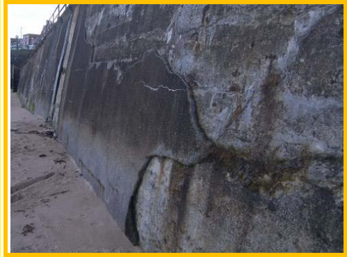
Continued loss of concrete encasement and corrosion of reinforcement mesh.
