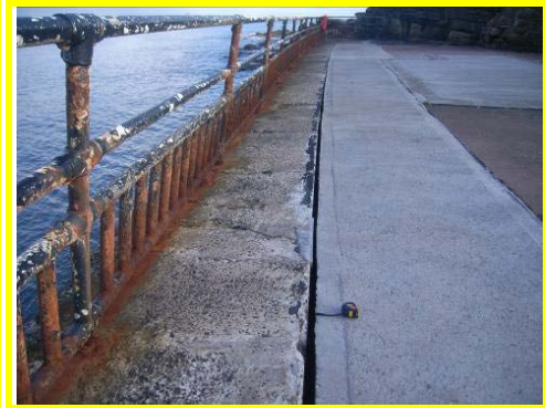
Wide gap between coping and surfacing at south end.
