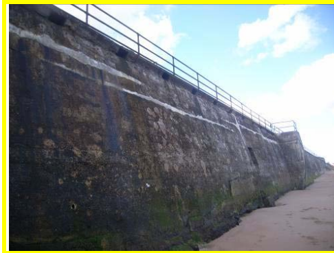
Recent repairs to horizontal cracks along upper section of sea wall at south end of Whitley Sands.
