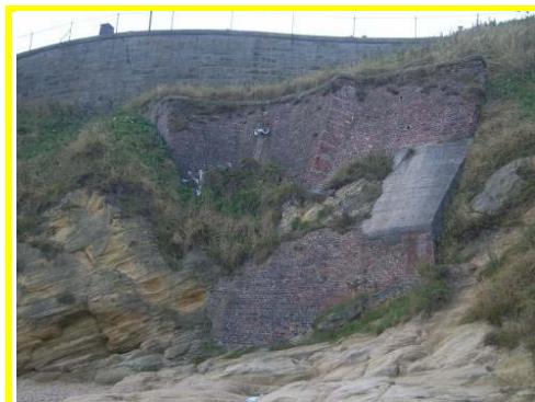
Masonry retaining wall at north side of Cullercoats Bay in fair condition.
