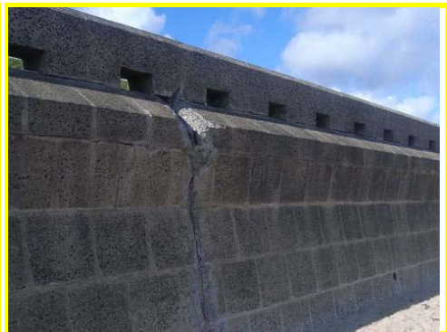
Gaps and missing mortar along the coping.
