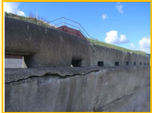
Cracking in render along cope of seawall.
