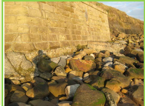
Concrete toe apron in need of repair.
