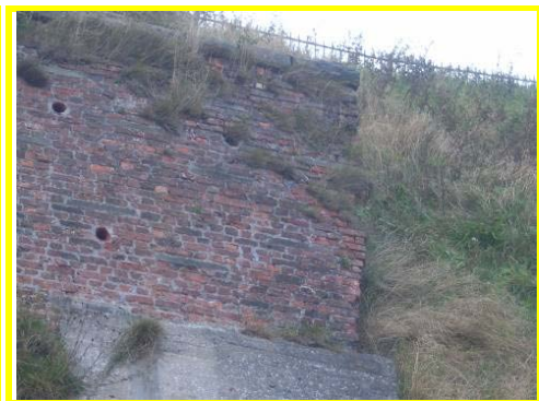
Missing mortar and gaps between bricks in upper wall.
