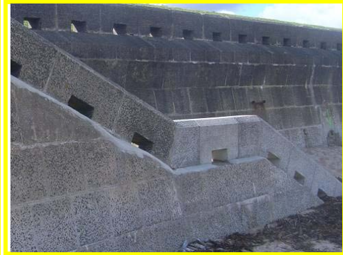
Repairs to some cracks along in Whitley Links Sea Wall good condition.
