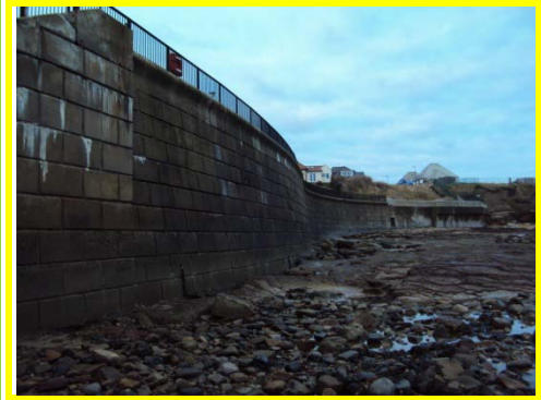
Concrete blockwork wall with local undermining to the toe.
