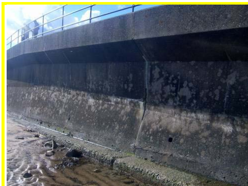
Low beach levels and exposed toe along the Trinity Road seawall.
