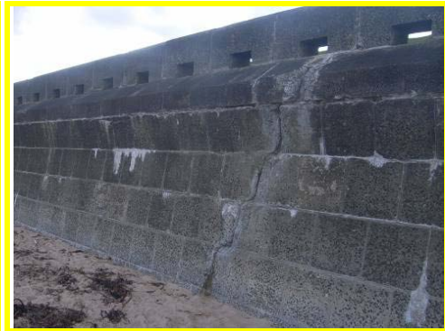
Diagonal crack through blocks south of Rendezvous Cafe.
