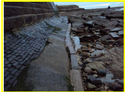
Apron to blockwork wall with signs of movement.
