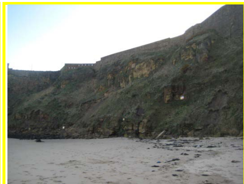
Signs of movement and slippage in vegetated cliff.
