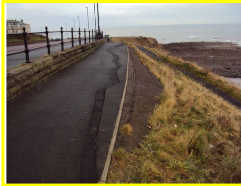
Cracking in upper slope.
