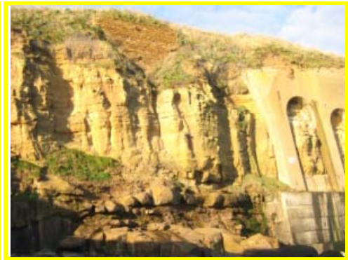
Some signs of slippage in the upper vegetated cliffs.
