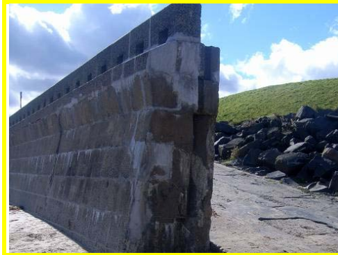
Repairs to some cracks along in Whitley Links Sea Wall good condition.
