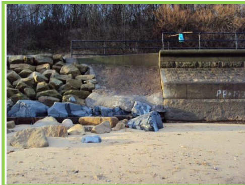
Remedial works at eastern end of revetment at Fish Quay in good condition.
