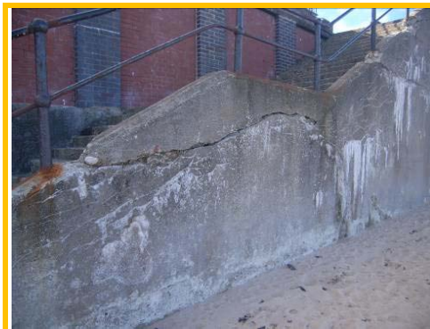
Cracks and abrasion at the access steps of the seawall.
