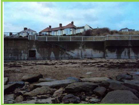
Concrete recurve wall and steps, steps have signs of abrasion.
