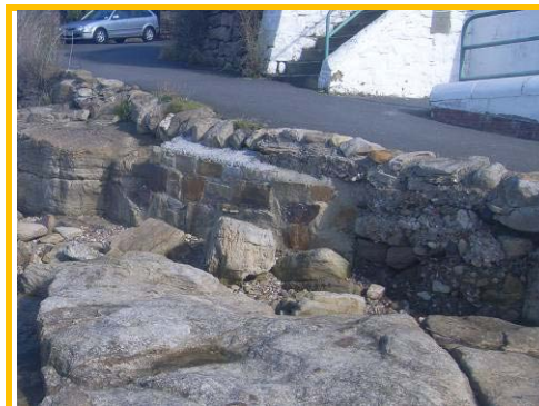
Missing masonry blocks and voids in low masonry wall at access ramp.
