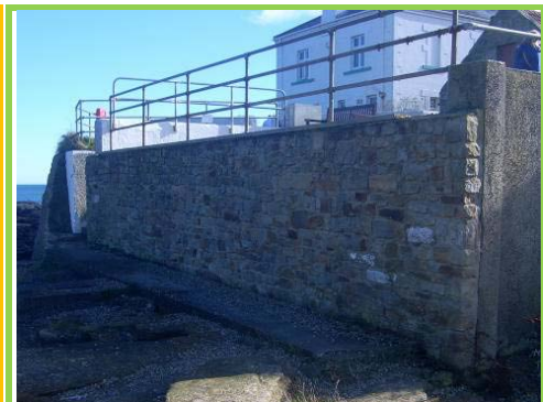
Void beneath masonry wall on north side of island has been filled.
