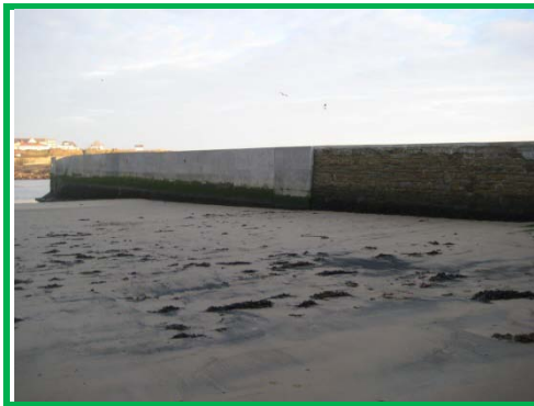
Leeward face of Cullercoats south pier with recent concrete repairs.
