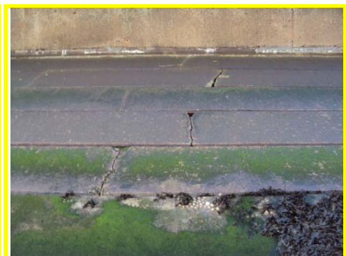
Cracking in panels and gaps at joints evident throughout
