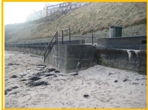
Handrailing missing to access steps.
