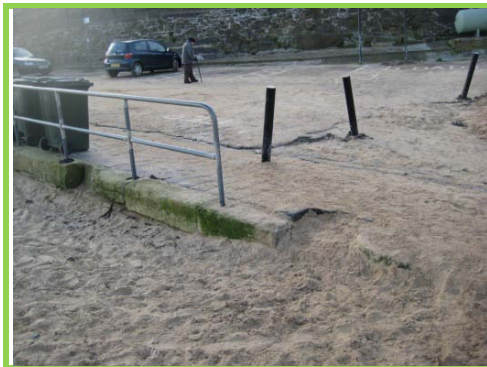
Missing coping and blocks to access ramp.
