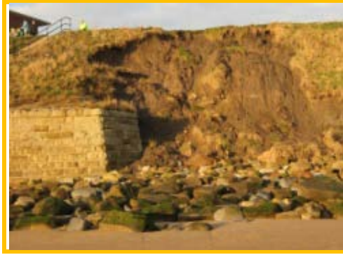
Slumping of cliffs adjacent to the masonry wall at Tynemouth Longsands.
