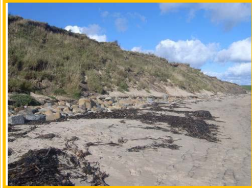
Cliffing evident along the top of the soft earth cliffs and boulder toe.
