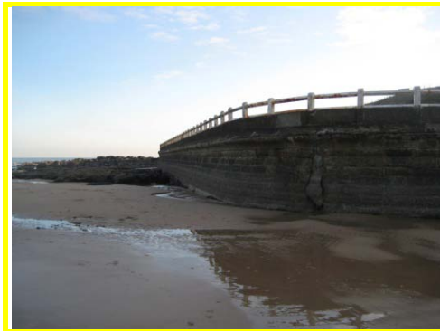
Damaged repair with concrete infill coming away.
