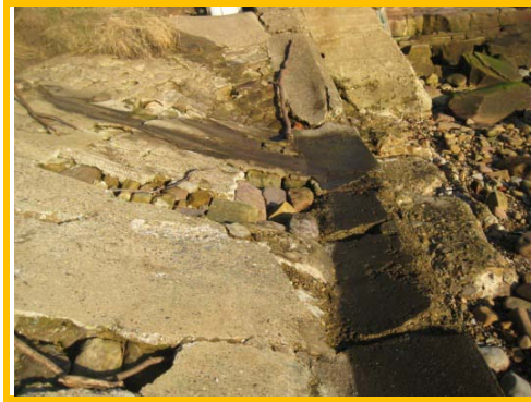
Failing revetment at Sandy Goit
