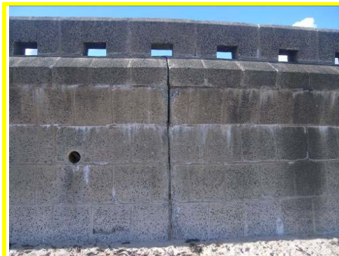
Full height gaps and abrasion in the wall at construction joints.
