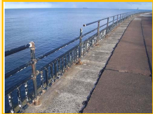
Missing section of hand railing at central section of wall.
