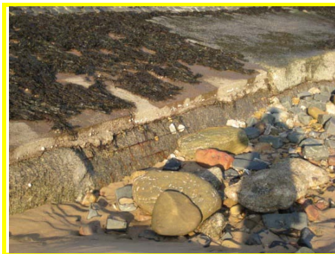
Abrasion at toe with exposed reinforcement
