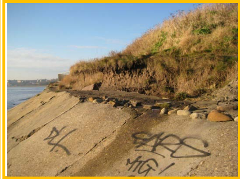
Erosion to upper slope
