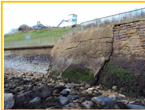
Spalling concrete render to masonry wall at Sandy Goit.
