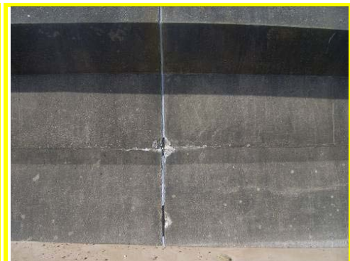
Spalling at some concrete joints and new sealant.
