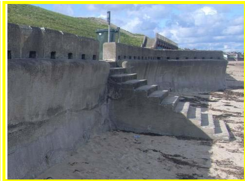
Damage along base of concrete steps no observed due to high beach levels.
