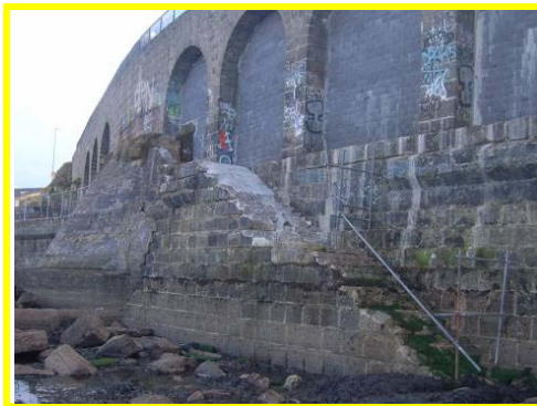
Dilapidated access steps are close and now redundant due to blocking up of arches.
