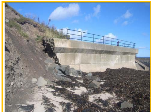
Continued outflanking at south end of wall and displacement of armour.
