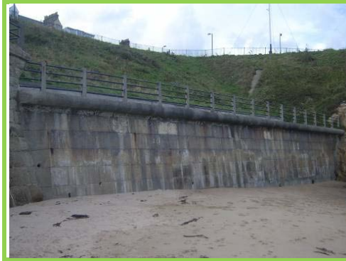
High beach levels along the seawall on the south side of Cullercoats Bay.
