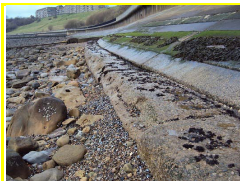
Abrasion to concrete toe of seawall at Knotts Flats.
