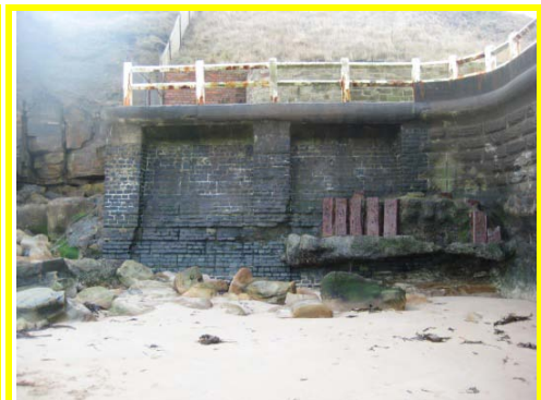
Wall at southern landward tie-in of Tyne Pool with apron undermined.
