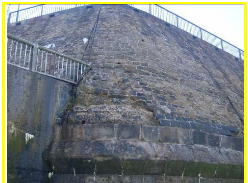
Section of missing brickwork at south end of upper sloping masonry wall.
