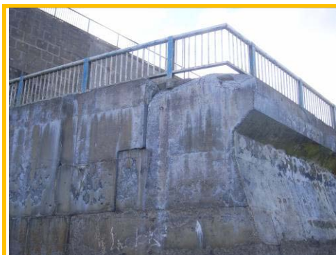
Missing section concrete along the crest has undermined one hand railing post.
