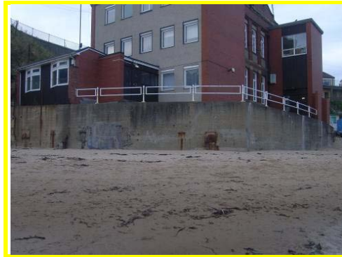
The concrete wall fronting the Dove Maritime Laboratory is in fair condition.
