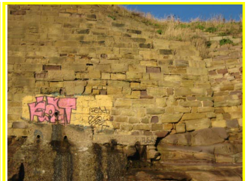
Gaps and cracks in mortar joints
