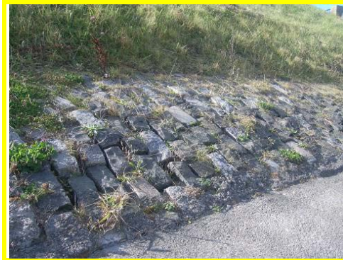
Vegetation growth and some gaps between blocks along revetment.
