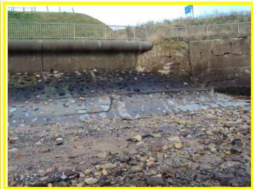
Cracking in pitched stone revetment
