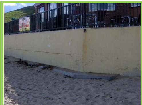
High beach levels covering exposed timber piles and undermining of wall.
