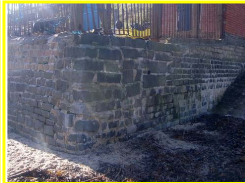
Some gaps and missing mortar in masonry blocks at north end of boatyard.
