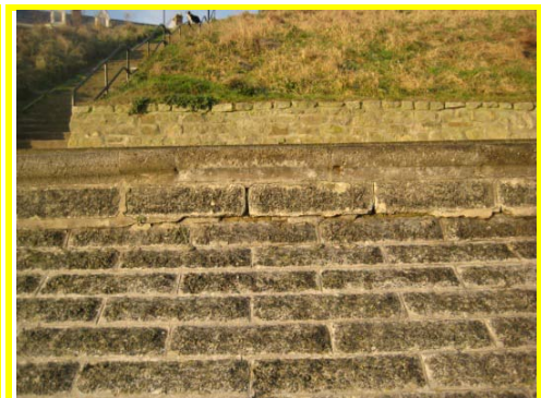
Localised damage to crest of masonry revetment with gaps in joints leading to cracking.
