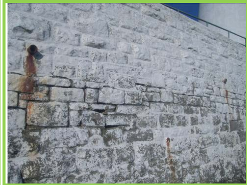
Minor loss of mortar to high masonry wall on east side of island.
