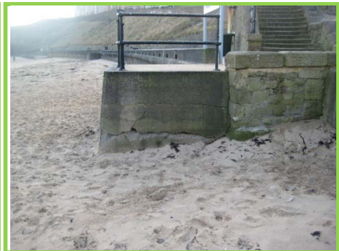
Cracking to concrete access steps
