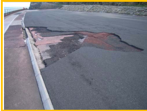
Damage to asphalt surfacing and missing kerbing at south end.
