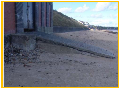
Cracks and gaps beneath the access ramps.
