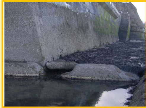
Voiding and undermining of toe apron at south end.
