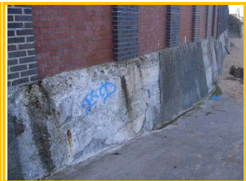
Abrasion and spalling of concrete encasing along the toe.
