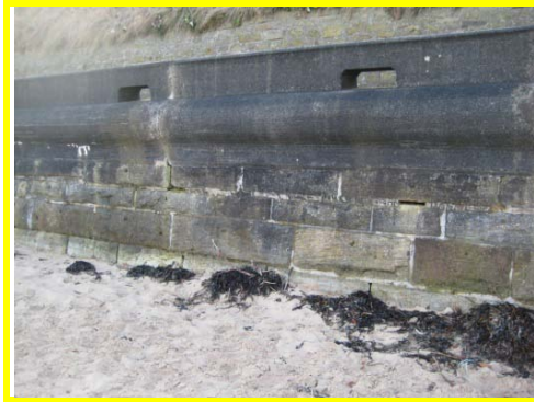
Missing mortar between joints.
