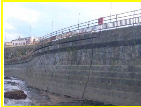
Missing mortar and gaps beneath coping at Southern Lower Promenade.
