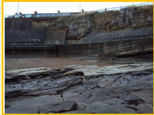
Southern wall and access ramp is locally in poor condition.
