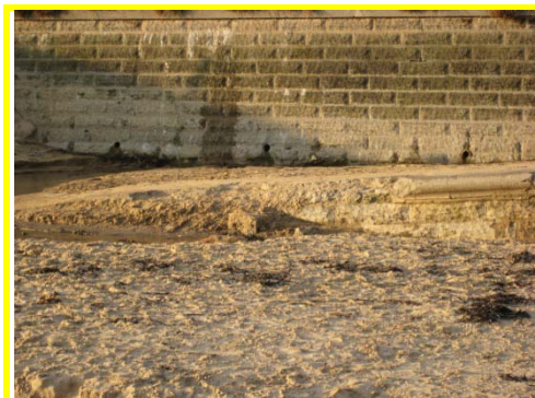
Spalling to concrete access ramp.
