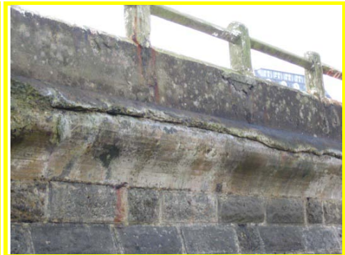
Abrasion and spalling to wave return wall.
