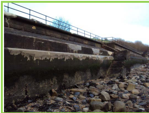
Heavily abraded access steps with patch repairs evident in foreground
