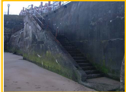
Missing lower post and hand railing at access steps.
