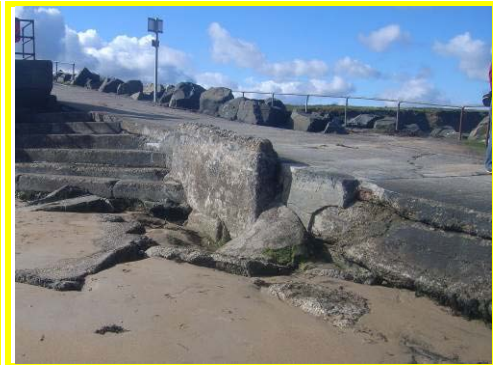
Some undermining of causeway but not currently cause for concern.
