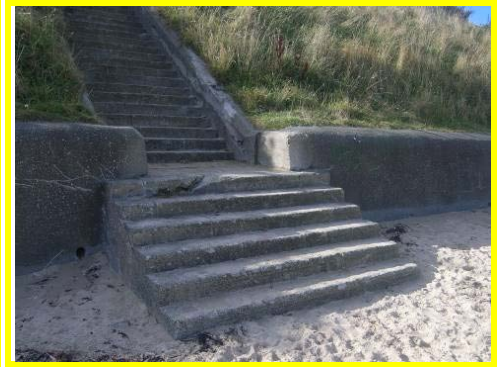
Cracks and spalling in concrete at the steps.
