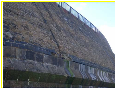
Section of missing brickwork at centre of upper sloping masonry wall.
