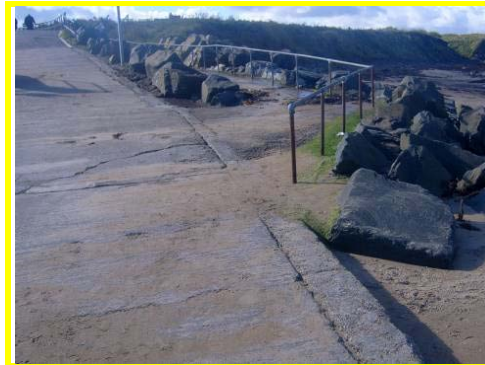
Cracks in the causeway to St Marys Island.
