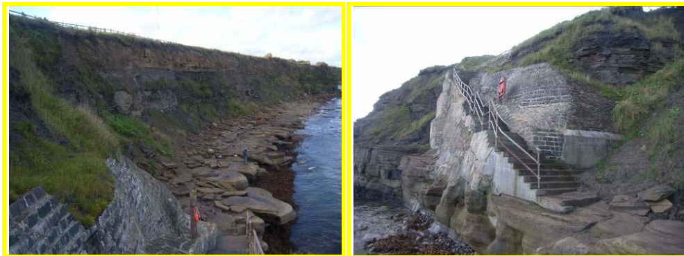
Rock falls and cliffing along high cliff and Hartley Cove.
