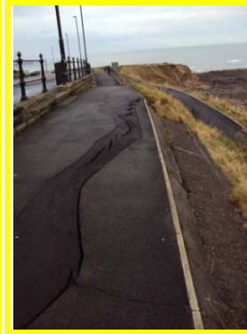
Movement at repaired cracks.
