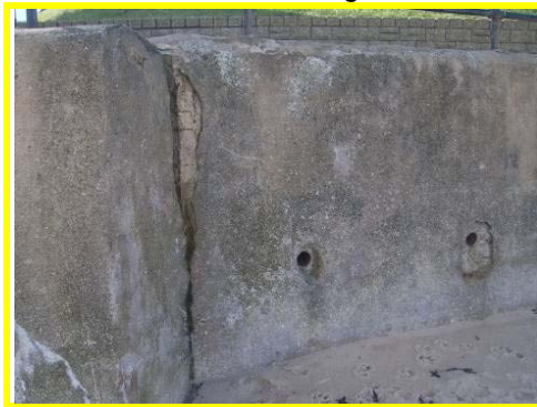
Spalling of concrete render and exposed rebar at south end of seawall.
