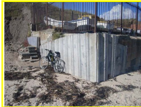
Repairs at south end of boatyard on Whitley Sands in fair condition.
