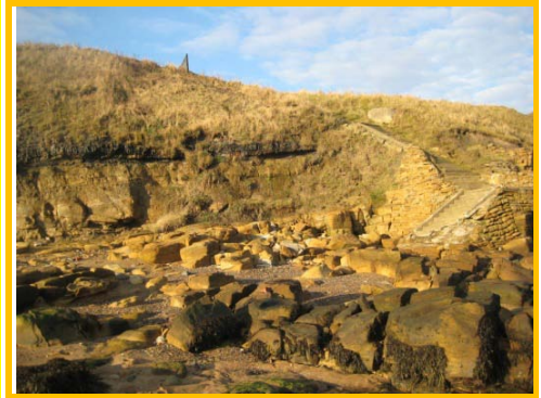
Heavily abraded access steps.
