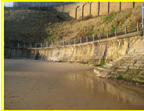
Curved sea wall in Kind Edwards Bay in fair condition.
