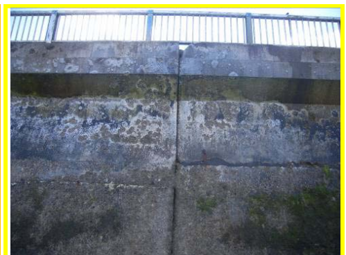
Missing sealant from construction joints.
