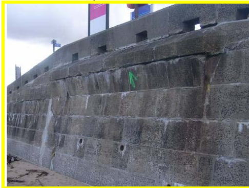
Gaps beneath the cope along the ramp at the Rendezvous Cafe.
