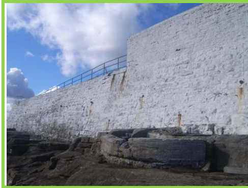
Masonry wall on east side of island well founded on rock foreshore.
