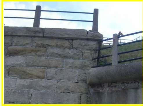
Movement and cracking between blocks at the north end of the high wall Section.
