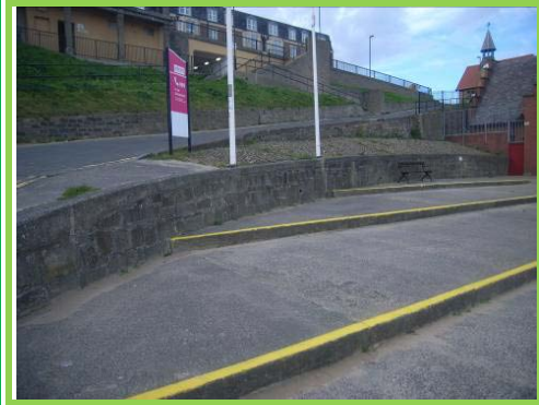
No apparent cracks or gaps in masonry wall at back of stepped apron.
