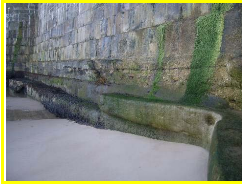
Abrasion at the toe of the straight section of seawall
